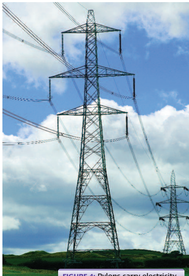
FIGURE 4: Pylons carry electricity wires overhead for safety.
