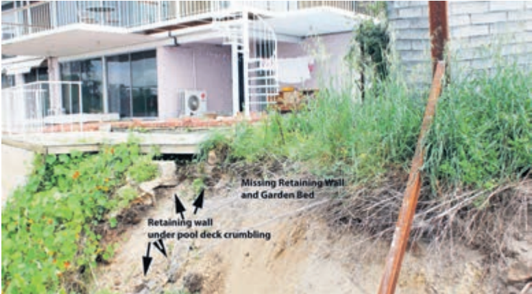
Mosman Park council says the loss of Anka Visscher's garden and retaining wall during construction of the Hughes mansion is a civil matter.
